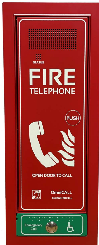
Figure 1.5 – Typical Combined Disabled Refuge / Fire Telephone
