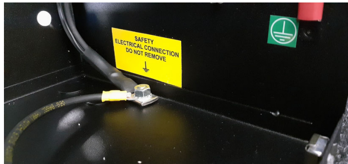
Figure 3 · Disconnect ground cables from star point (if required) to prevent damage
